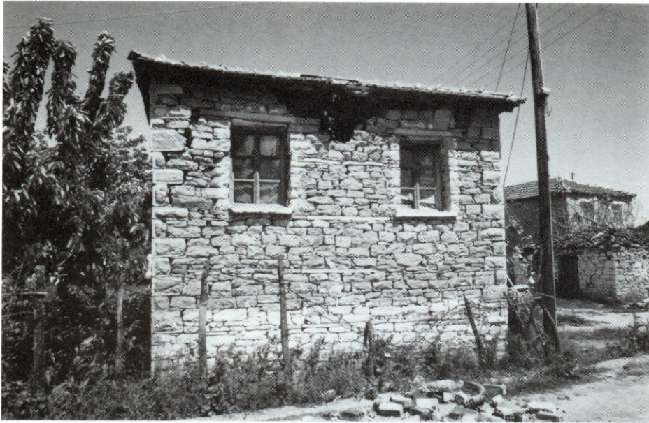
Figure 4 —Typical old house of the region reinforced with wooden beams. Houses of the same type but without the wooden beams suffered much more damage or collapsed.
