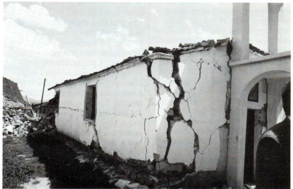
Figure 5 —The damaged church in the village of Knidi. The cracks are typical of the strong vertical component of the ground motion.
