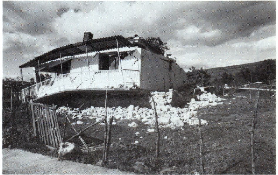
Figure 1 —Typical damage to the buildings in the region struck by the earthquake.
