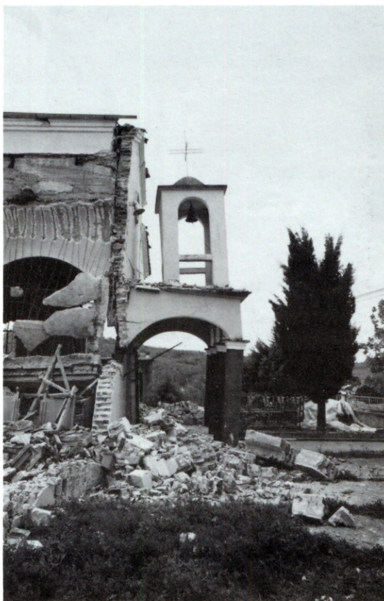
Figure 6—A view of a damaged church in the village of Kendron.
