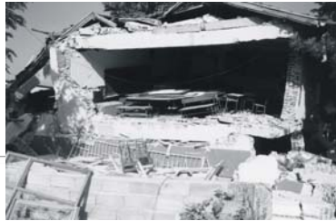
Figure 5: A collapsed school building, made of supporting brick masonry, within the subsided block.
