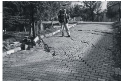
Figure 3: Partial view of the southern fault segment, with vertical (normal) and horizontal (right-lateral) offset components, marked by the dislocation of flagstones. At least five breaks are visible.
